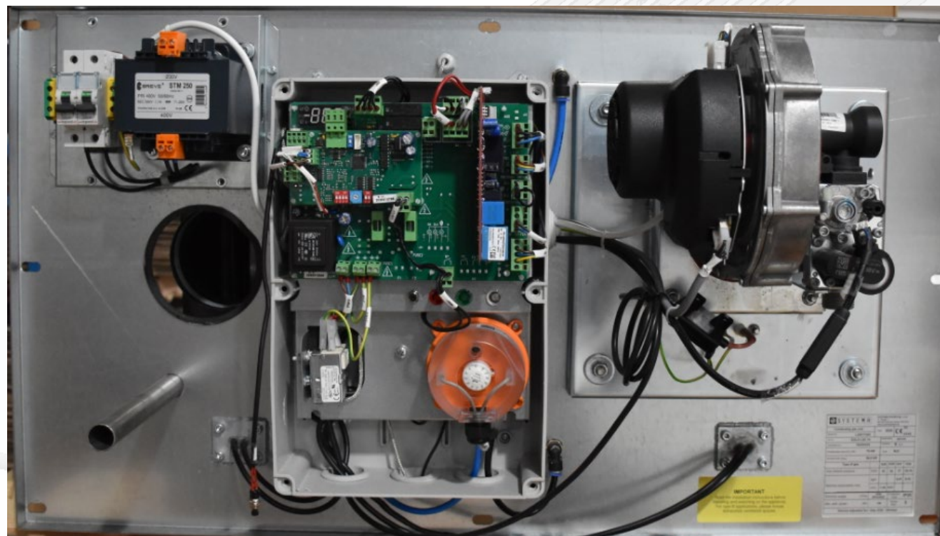
View of heat exchanger gas unit – E Baltic C box
